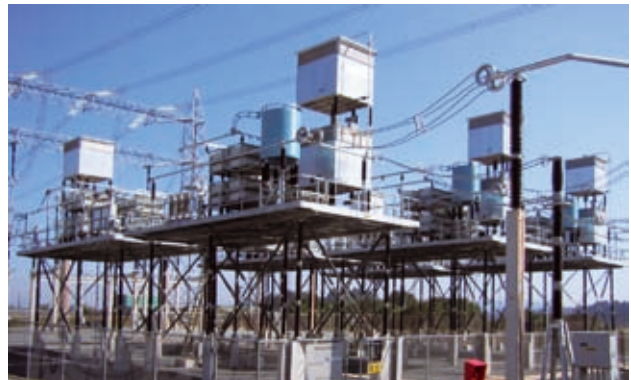
Fig. 5 Series capacitor bank, 765 Mvar, 500 kV - 60 Hz at Ibiúna substation in Brazil.
