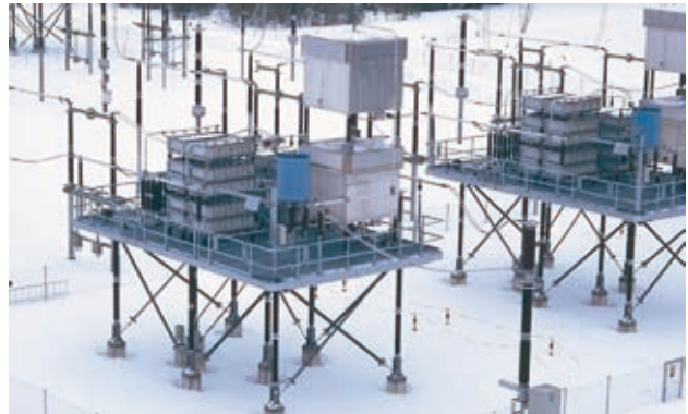
Fig. 4 301 Mvar 400 kV - 50 Hz series capacitor bank at Kemimaa substation in Finland.
