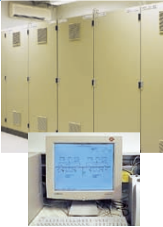
Fig. 6 Typical arrangement of the control cubicles and HMI in the control building.
