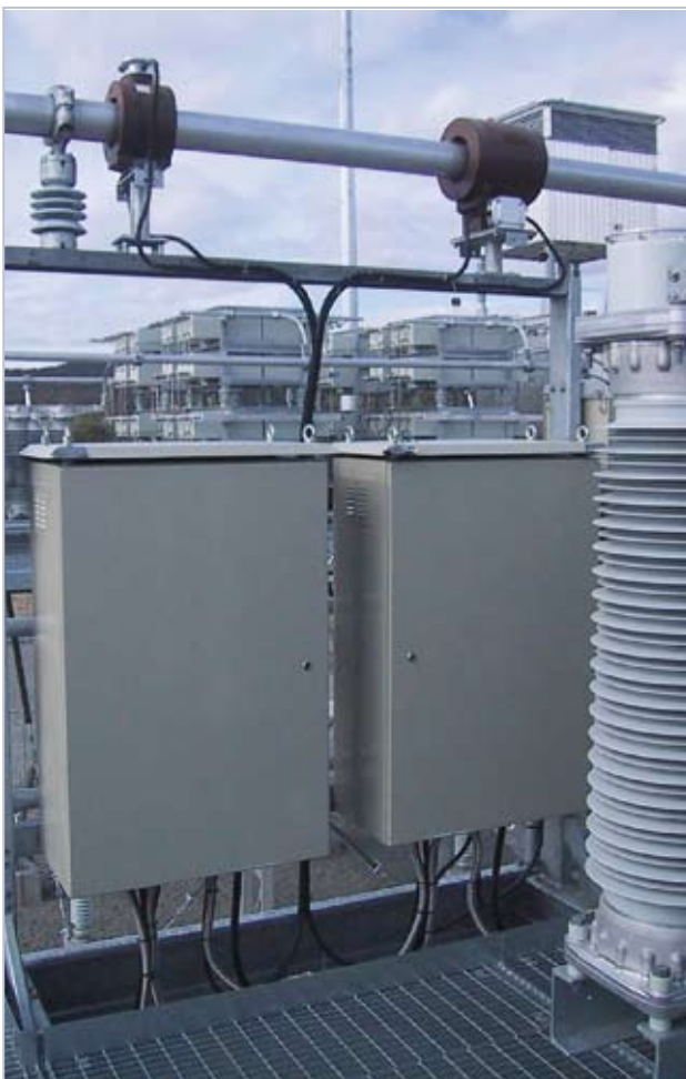
Platform cabinets transmit measurements to the control and protection system on the ground level.
