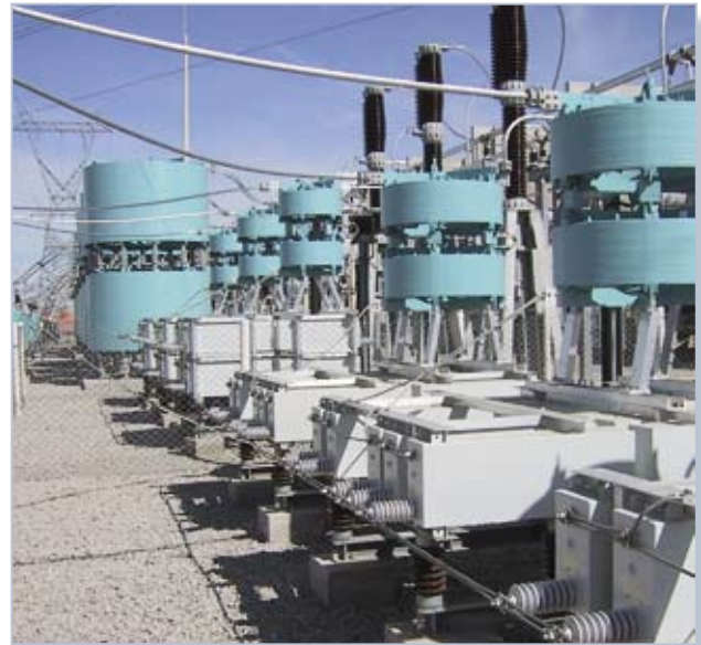
-60...+100 Mvar, 345/15 kV, 60Hz, Campos, Furnas Centrais Elétricas SA, Brazil
