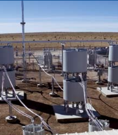
Thyristor control reactors.
