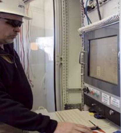
A member of Tri-State's safety personnel conducts testing of the new system.
