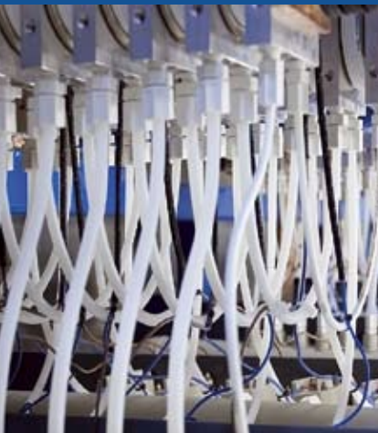
The new thyristors and cooling system.
